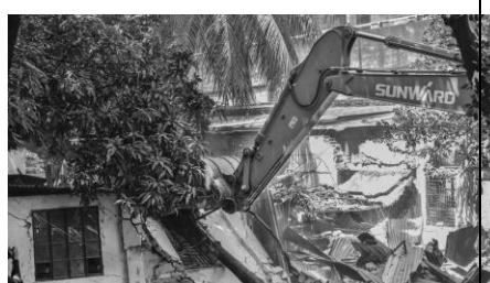
Figure 5. Bangladesh Railways demolished 250 illegal structures from Dhaka's Shahjahanpur Railway Colony on September 17, 2019.
