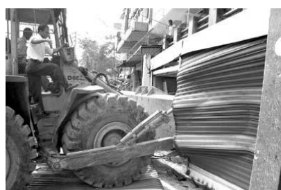
Figure 8. An illegal portion of Genetic Plaza at Dhanmondi, Road No-27, bulldozed by RAJUK
