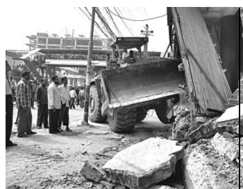
Figure 9. RAJUK knocked down illegal structures at Purana Paltan in Dhaka
